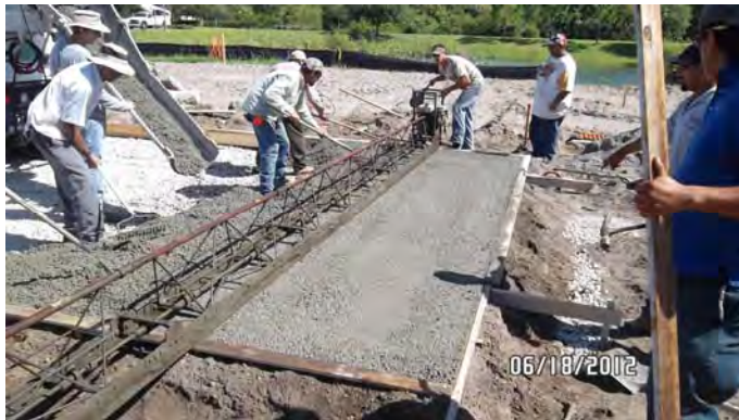
Installing Pervious Concrete Parking Space at SCAT Park and Ride at North Port City Center
