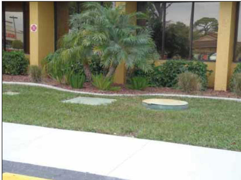
Figure 4. Private Lift Station – Provision Eye Center.
