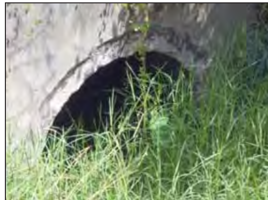
Figure 103. Stormwater Pipe from DP38-184 to Vault.
