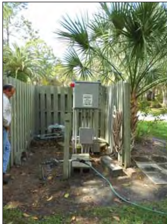
Figure 44. Gasparilla Condominium – Private Lift Station.
