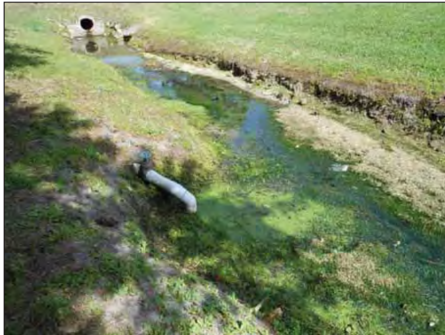
The stormwater pond overflows into the ditch; irrigation pipes observed (foreground).
