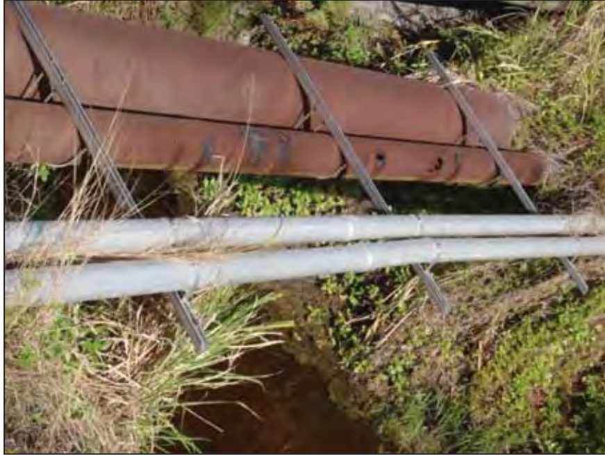
Figure 7. Aerial Crossing – Rusted out old raw potable water lines across open stormwater canal.
