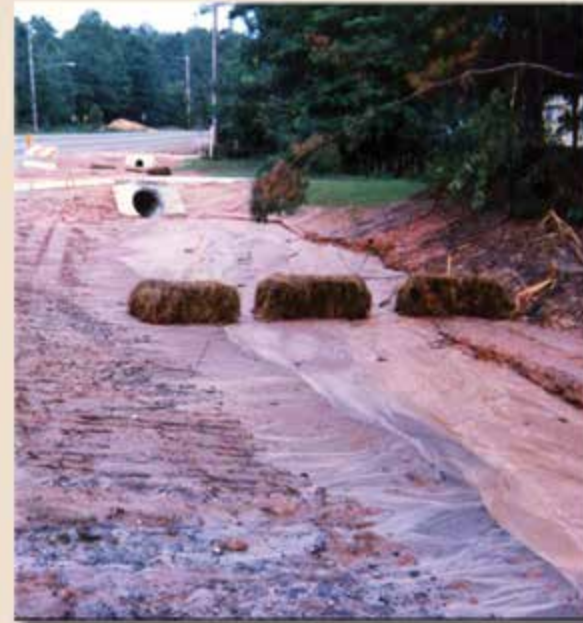
Example of improperly installed erosion control devices and resulting erosion
