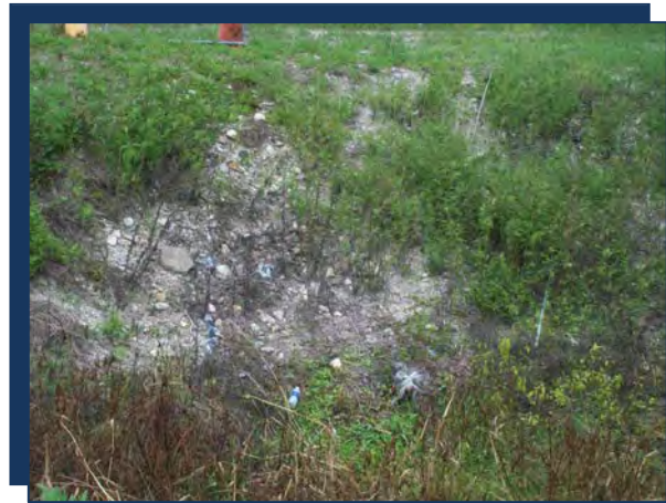
Photo: AC06 General Bank Condition
