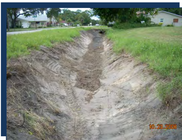
Photo: AC08 Denuded Swale (Looking West)
