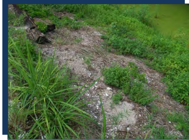
Photo: AC01: General Bank Condition
