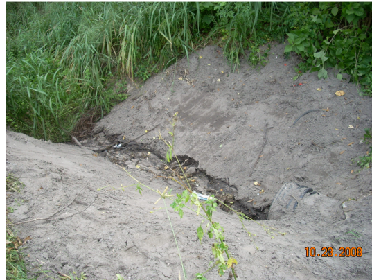
Photograph 4 Erosion at Outfall Pipe
