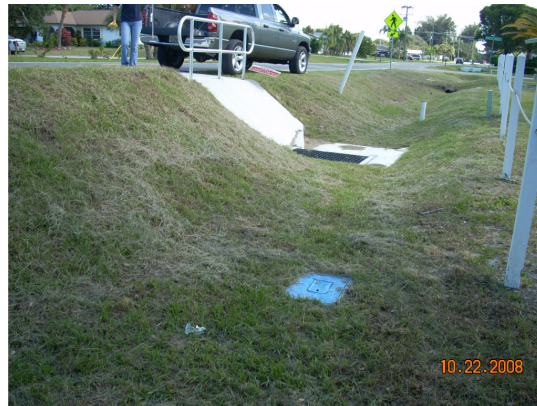
Photograph 1 Grass Clippings Lining Drainage Swale
