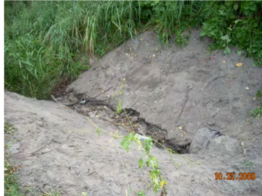
Photograph 4 Erosion at Outfall Pipe
