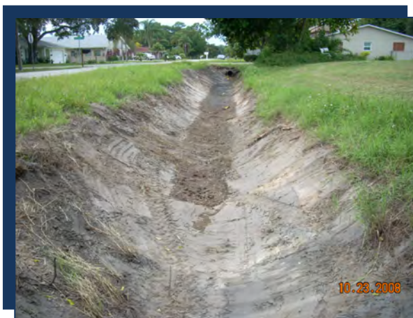
Photo: AC08 Denuded Swale (Looking West)
