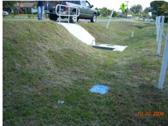
Photograph 1 Grass Clippings Lining Drainage Swale
