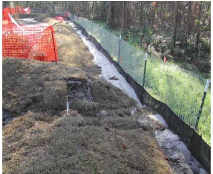
During construction, block off the shoreline with a temporary construction fence to prevent damage from heavy equipment and construction activities.
